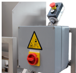
Operator/control panel with emergency stop.
